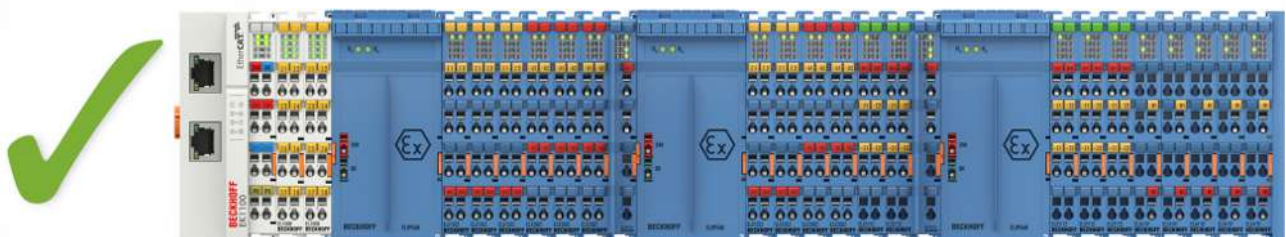
Fig. 9: Valid arrangement - multiple power supplies by ELX9560, each with an upstream ELX9410.
